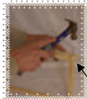
STEP 6: Drive two nails in, at each end of the top bar as shown.
