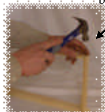
STEP 7: Nail into the non-wedge part of the frame, slanting well into the top bar.
